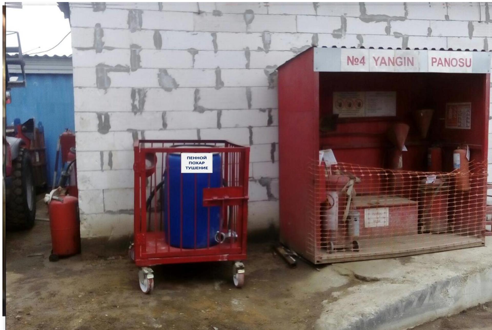
Broken Fire Hydrant System
